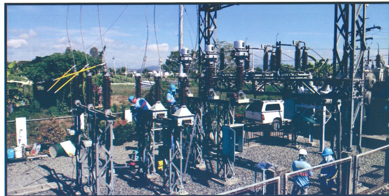
UPDATED 20MVA SUBSTATION MALAPAT, CORDON, ISABELA
