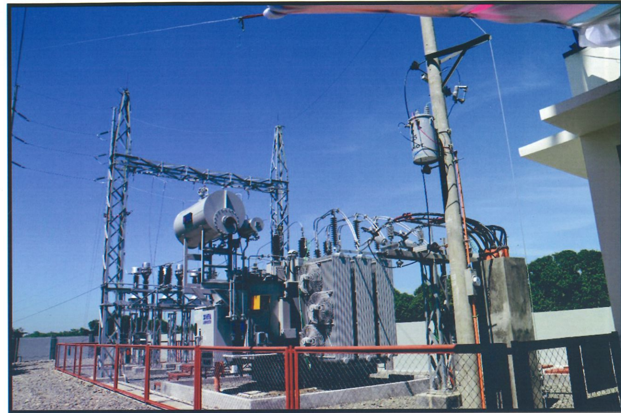
20MVA SUBSTATION SAN FERMIN, CAUAYAN CITY, ISABELA
